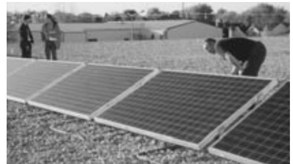
Two-kilowatt photovoltaic system installed on the roof of Waunakee High School.
