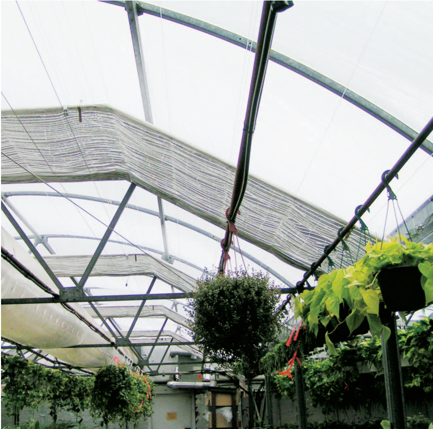
Moveable insulated curtains can reduce heat loss from 20 percent to 70 percent depending on curtain material.
