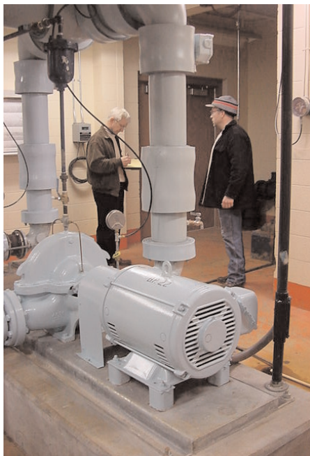
An energy assessment is taken at the Fond du Lac, Wisconsin, Water Treatment Facility.
