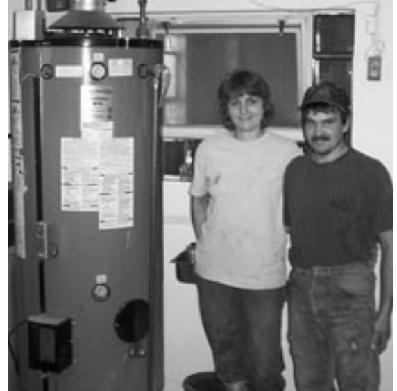
The new water heater installed at the Behnke's farm has reduced utility costs and improved productivity.
