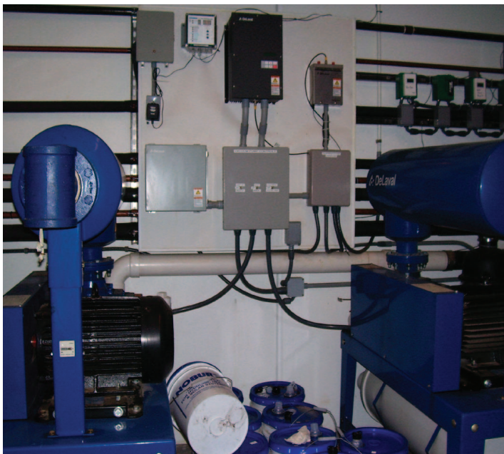
The variable speed vacuum pump system maintains exact vacuum specifications and minimizes energy use from the vacuum pump.
