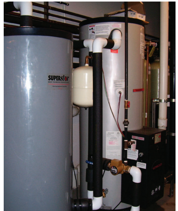
The heat recovery tank captures heat from the Griesen's refrigeration system. This heat is used to reduce their hot water energy use and expands the capacity of their water heater.
