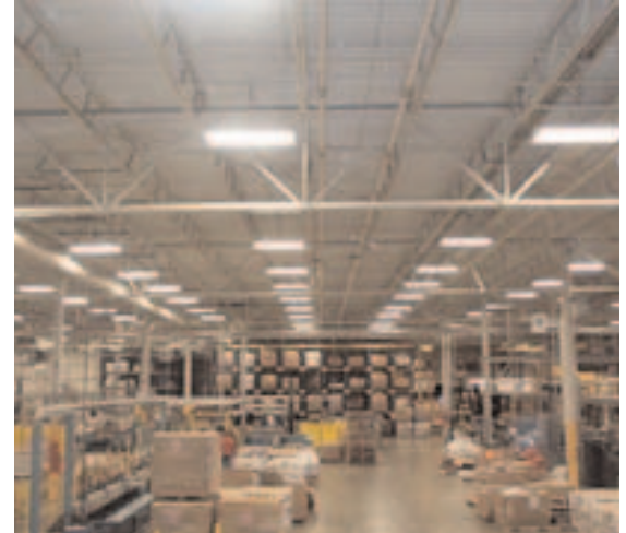
HIGHBAY FLUORESCENT LIGHTING
