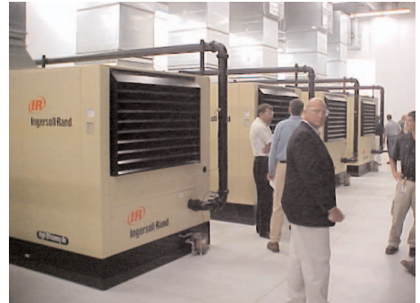
New Baseload Compressors
