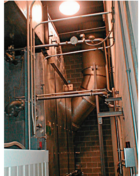
New condensing economizer and exhaust stack.
