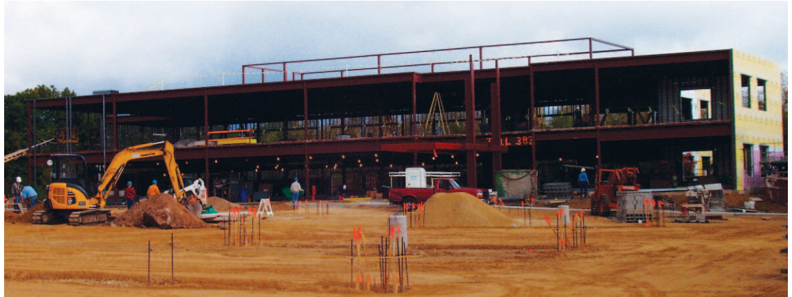
Achieving high performance starts in the design phase and continues through construction.
