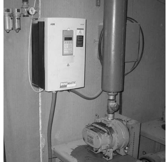
A typical variable frequency drive installation.
