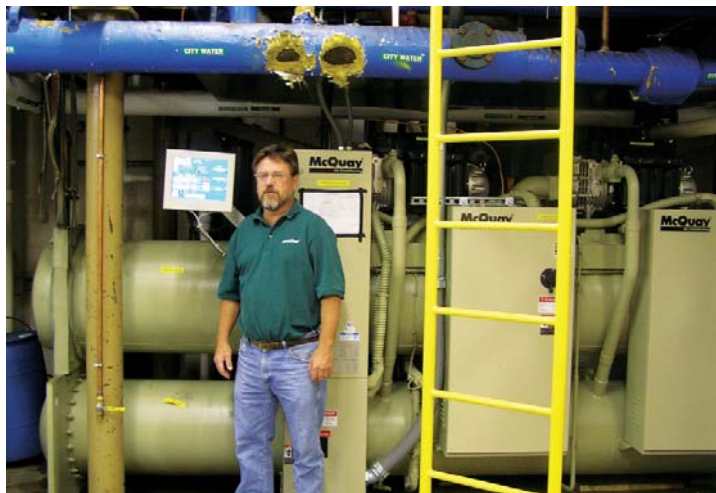
Frank Rushmann, Phillips Plastics Facility Manager, with new McQuay turbo core chiller with digital operator interface over right shoulder displaying current energy consumption.
