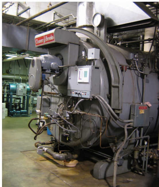
A burner upgrade and new controls saved the Siena Center $15,813 in energy costs during a one year period.
