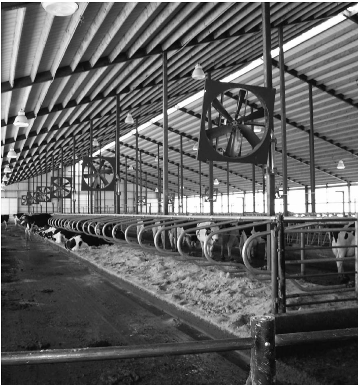
Optimal spacing and adequate fan capacities are necessary for an effective cow cooling system.
