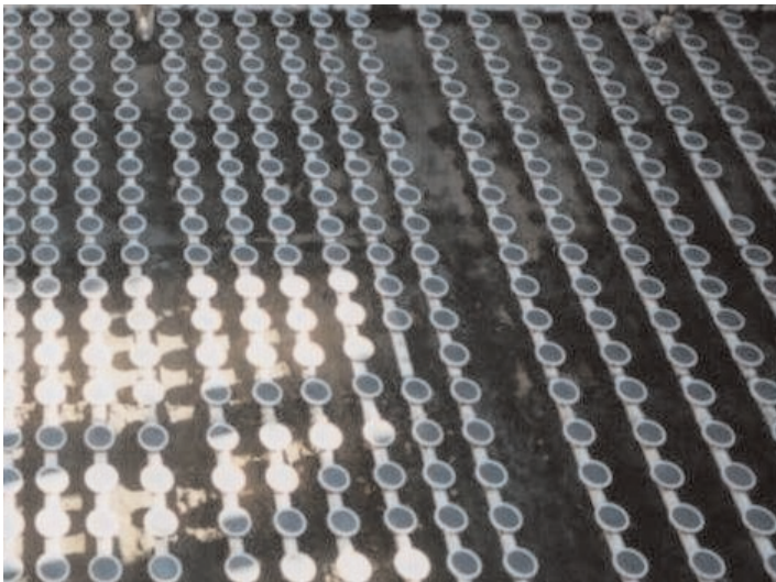
Fine Bubble Aeration, Sheboygan, Wis.
