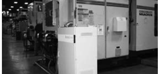
SyncroSpeed, a variable-frequency drive hydraulic control system, next to Xten's largest press.
