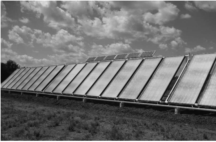
The panels provide about 18 percent of the brewery's annual hot-water needs.
