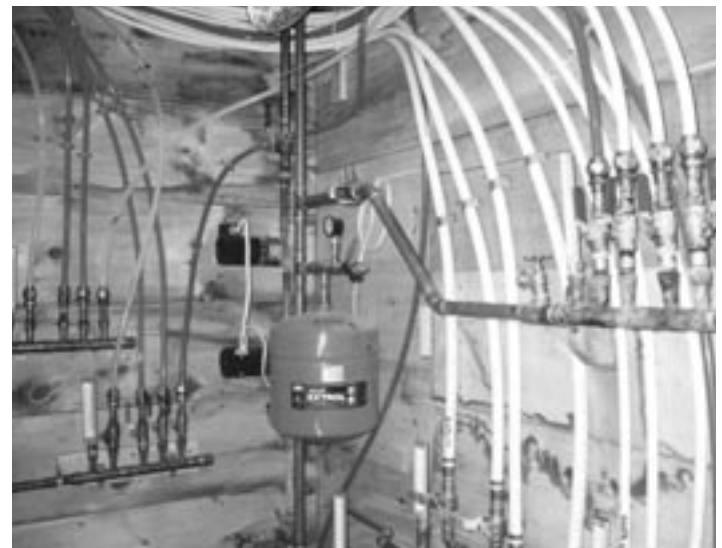
This photo shows the hot water piping in the Davenport's mechanical room. The home is divided into separately controlled heating zones, and each zone has its own loop of piping.
