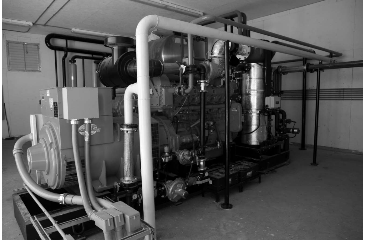
This engine generator uses biogas from manure digestion as fuel. The generator produces about 225 kW of electricity.
