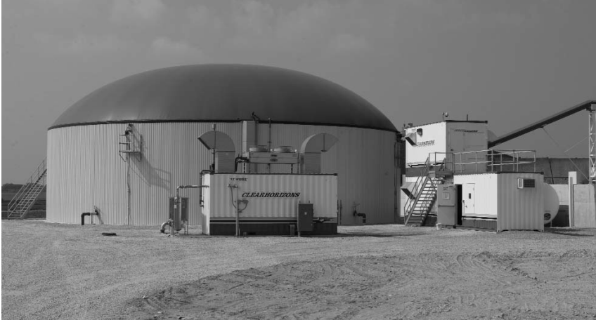
A complete-mix digester at the Crave Brothers Farm near Waterloo, Wisconsin also incorporates waste from their farmstead cheese facility which is located across the street from the digester.
