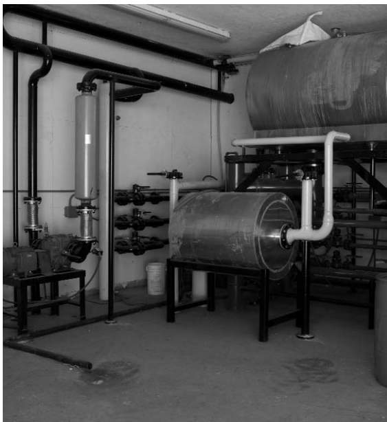
Heat exchangers like this one transfer heat from the engine generator to the digester in addition to the heating system for a barn and office.
