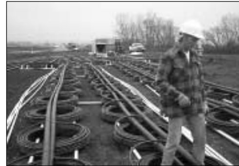
Preparing for loop assembly to be placed in the pond. Each loop equals one ton of HVAC.
