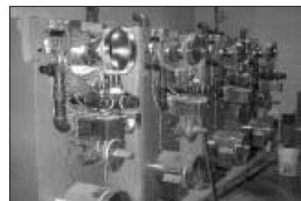
Photo below: 1.9 million BTU boilers.
