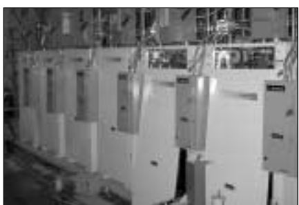
Photo below: Water to water heat pumps (14 total.)
