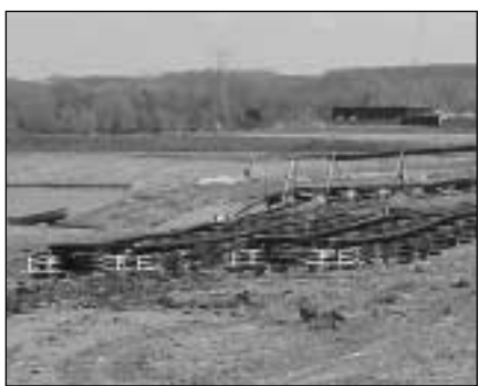
Series of loop assembly on shoreline. A total of 720 will be placed in the ponds.
