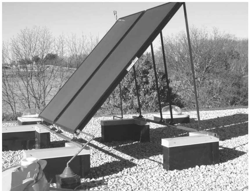
The solar thermal system on the Wisconsin Energy Conservation Corporation building will provide 40 percent to 45 percent of the hot water needed in restrooms, breakroom and fitness room showers.
