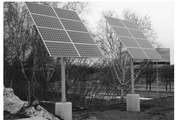
The Wisconsin Energy Conservation Corporation's solar system includes four small, attractive and highly visible "solar flags" located in the parking lot and on the grounds. Overall, the roof-mounted solar electric panels and the solar flags produce 19 kW of electricity.
