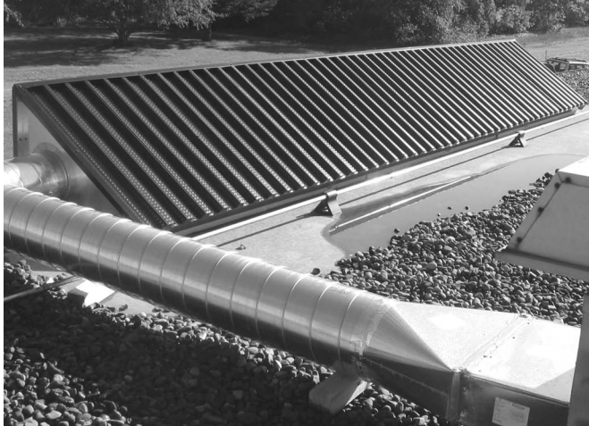
This SolarDuct® installation, the first in Wisconsin, augments the building's natural gas-fired heating system, saving energy costs.
