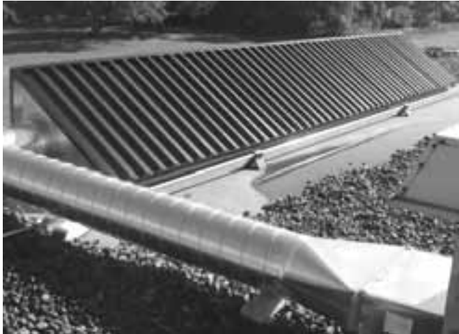
This SolarDuct® installation, the first in Wisconsin, augments the building's natural gas-fired heating system, saving energy costs.
