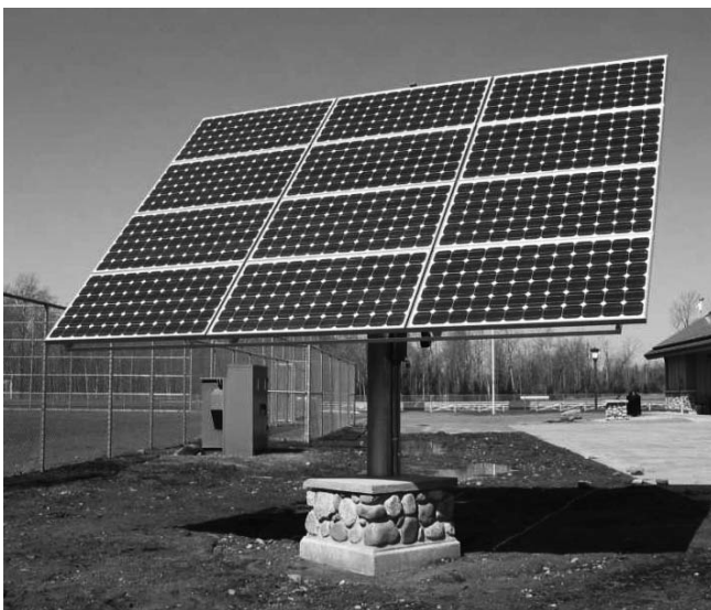
2.16 kW pole-mounted tracker solar electric system located on the grounds of the Conservation School in Land O' Lakes, Wis.
