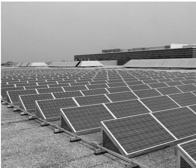
135 kW ballasted rack-mounted solar electric system located on the roof of the GE Health Care building in Waukesha, Wis.
