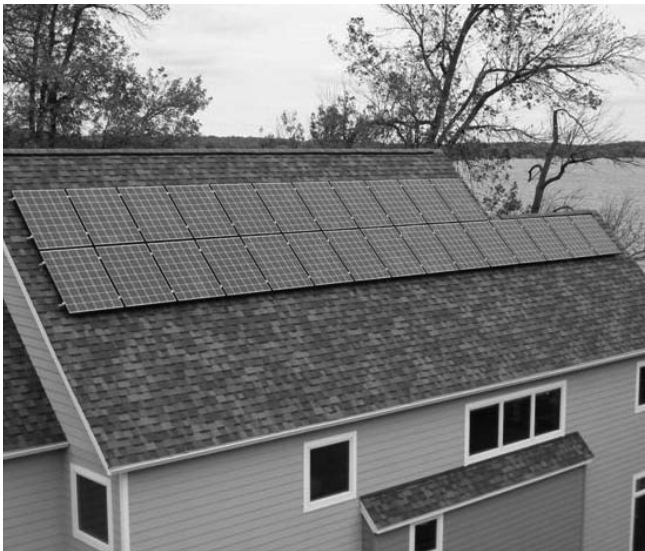
4.55 kW flush-mounted rooftop solar electric system located at a residential property in Middleton, Wis.
