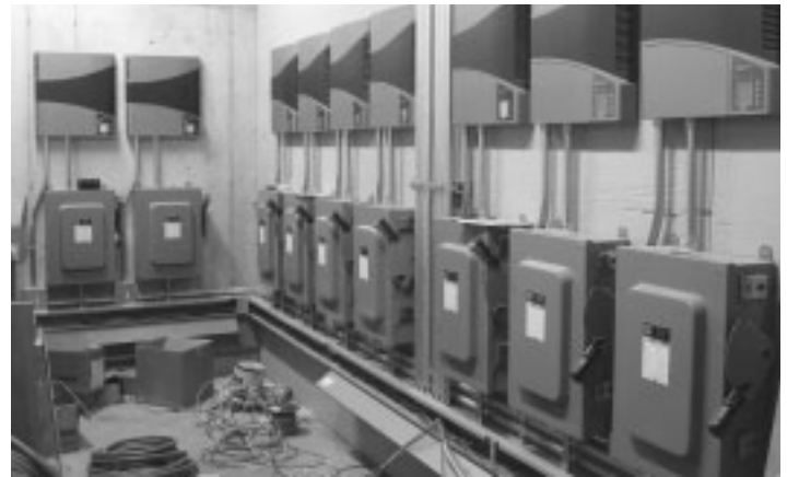
PHOTO: H&H SOLARELECTRIC
