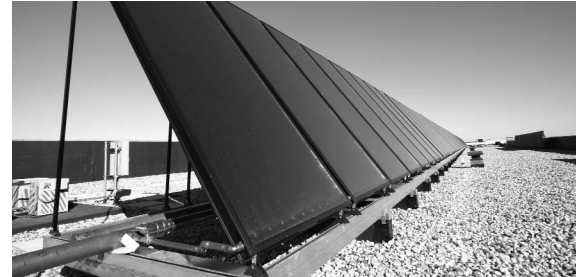
This impressive 104-panel solar hot water system atop the Kalahari Resort & Convention Center in Wisconsin Dells supplies the laundry facility with more than 3,000 gallons of hot water per day.
