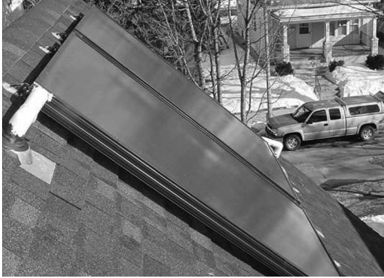
Solar collectors supply the home's new solar water-heating system.
