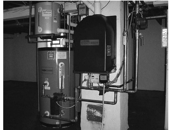
A high-efficiency boiler and solar thermal water-heating system replaced a 1960s-era hot water boiler (62 percent efficiency) and 0.52 EF natural-draft water heater.
