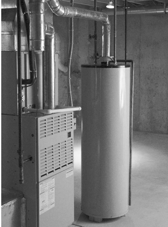
Atmospherically vented appliances, such as this water heater, should be direct-vented to minimize carbon monoxide exposure.
