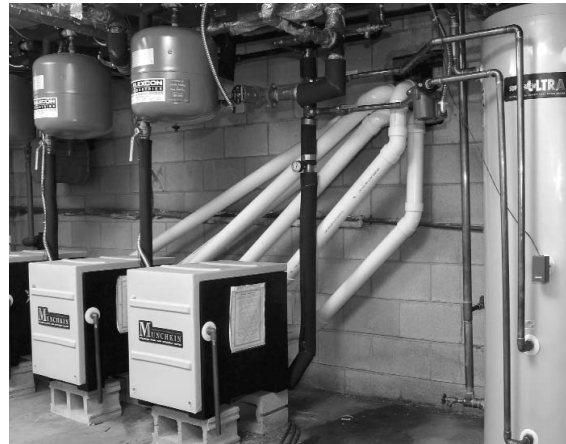
Updating to state-of-the-art boilers and sidearm water heaters at Grange-Allison apartments helped John Wirth save $54,000 in energy costs in just three years.
