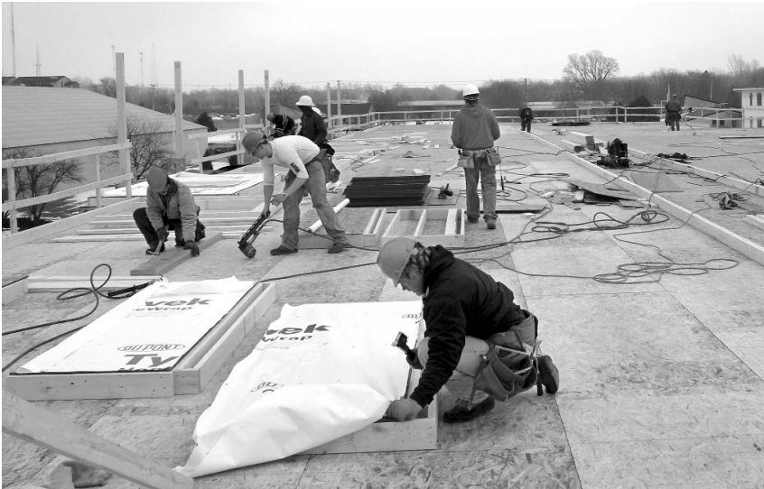
Attention to detail—from building orientation and insulation to energy efficient building materials and efficient HVAC equipment to the installation of renewable technologies—can spell the difference between an average property and an energy efficient, cost-saving, valuable new building.
