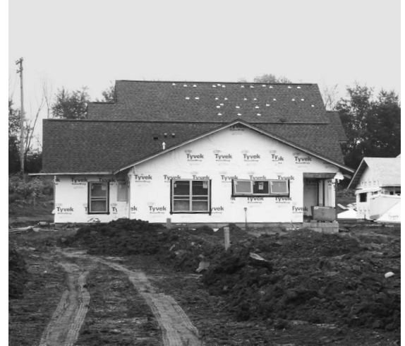
Troy Gardens' developers were able to work with Focus on Energy to take advantage of energy saving measures and building science principles.
