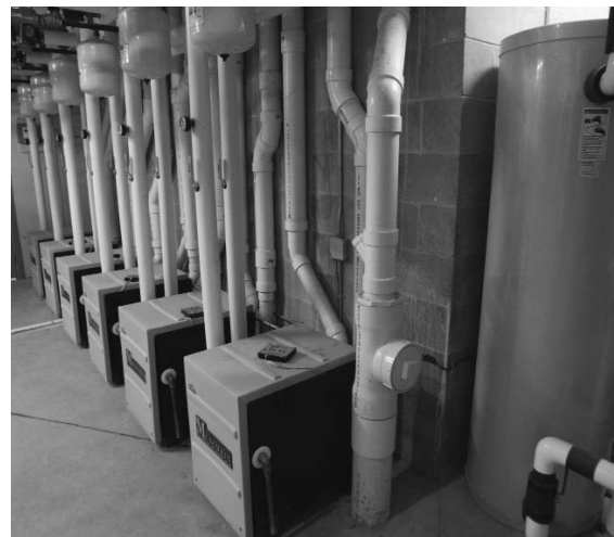
High efficiency Munchkin-brand boilers help heat water throughout the complex. The boilers only turn on when needed.
